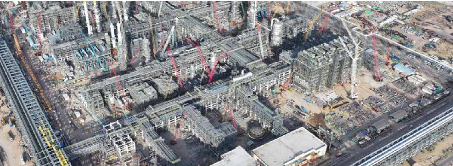
Dual Feed Cracker Block Unit (DFCU) for HRRL, Barmer, Rajasthan
